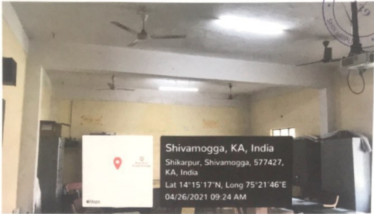
Led Bulb Facility in the Staff Room
