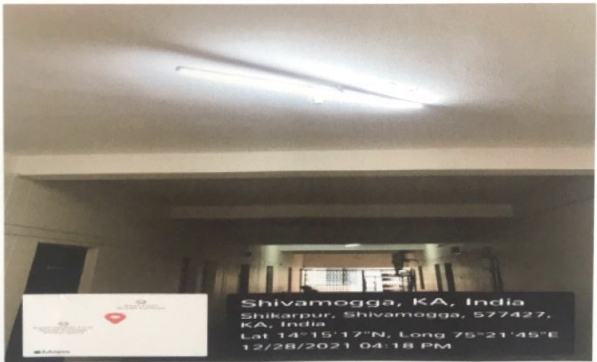
Led bulb facility in the corridor
