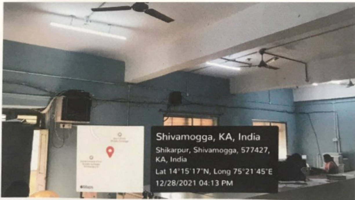
Led Bulb Facility in the Office
