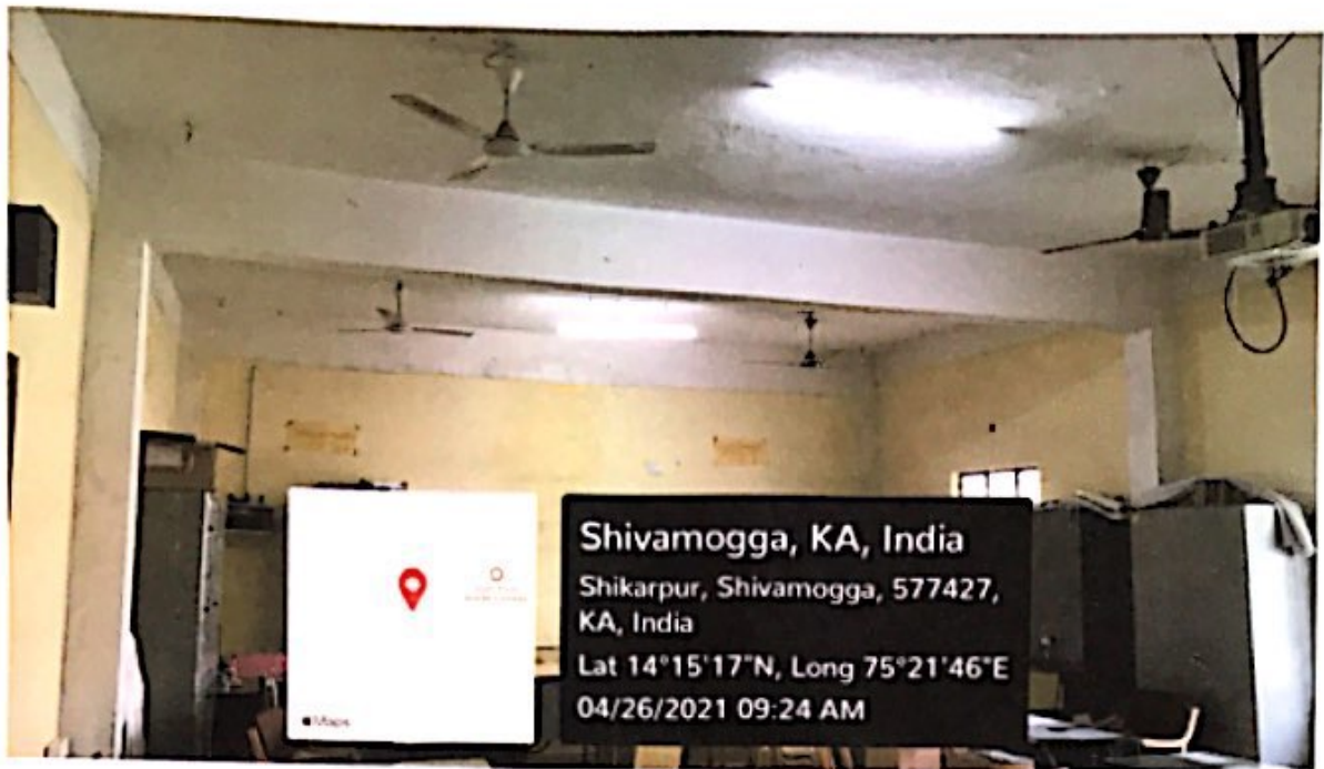
Led Bulb Facility in the Staff Room
